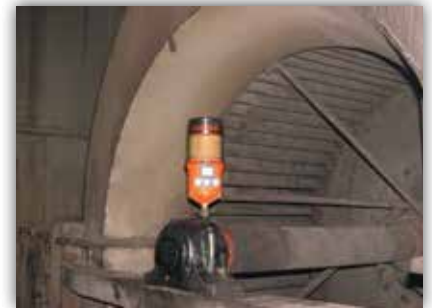
Grease lubricator installed on a blower fan
