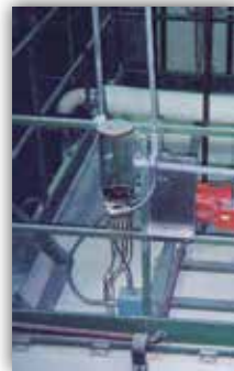
Gravity feed oiler on drying machine
