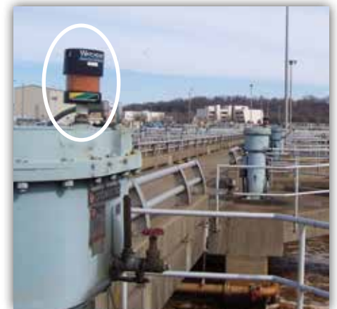
Watchdog Breather installed on a gearbox at a water treatment facility
