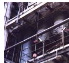
Catalyst hopper level gauges
