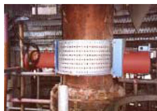
Nucleonic density gauge on reactor
